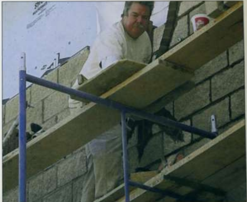
Skilled brick mason John Steele is reproducing the church logo in brick on each end of the facility. (Photo by Keith Kappes)
